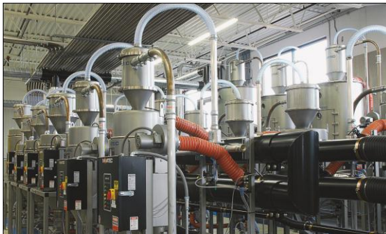
Dry air is circulated to each hopper through a closed-loop manifold.
