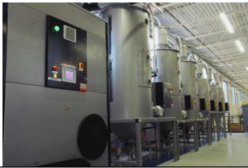
Central Dryer with Central Drying Hoppers
